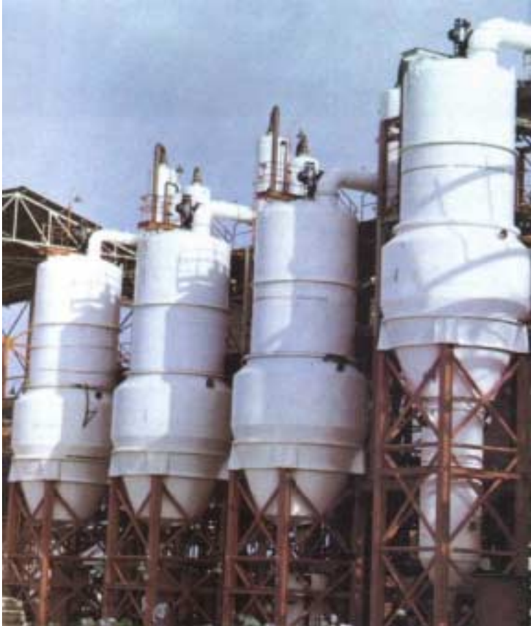
Left: Swenson Draft Tube Baffle crystallizer system for production of potassium chloride from Dead Sea brine.
