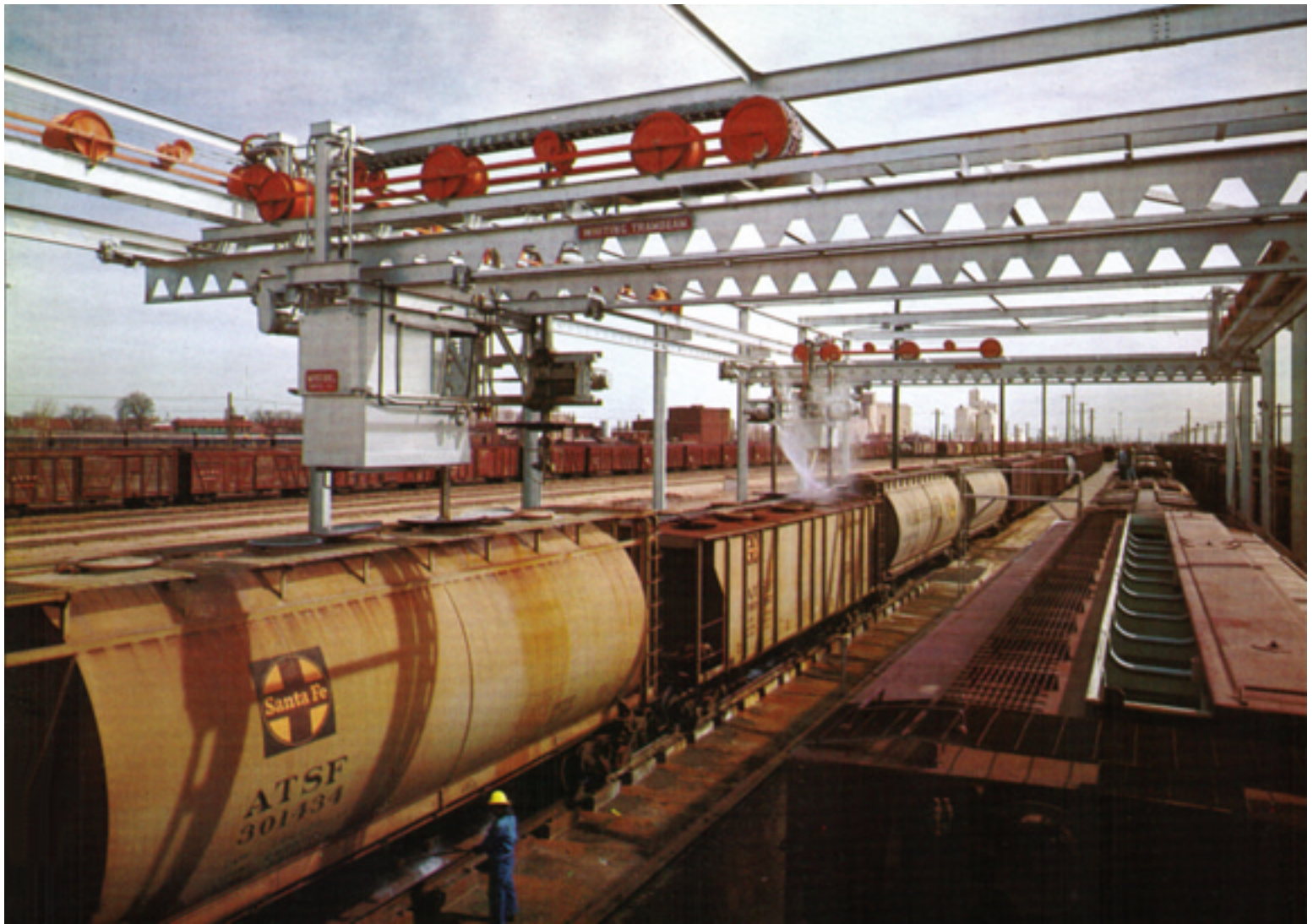
Whiting underhung cranes have lowered washing wands into first two cars visible on track at left. (Note escaping spray at top of second car.) The 48-car cut on track at right is being advanced in two-car increment by Whiting ROBOTS. Trolleys will traverse to wash cars on right track while cut on left is being advanced.
