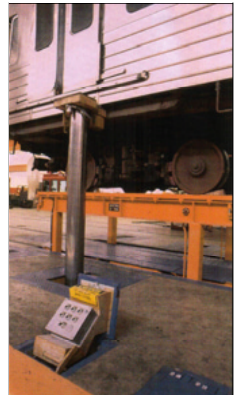
Body hoists support the car in a level position during truck removal.
