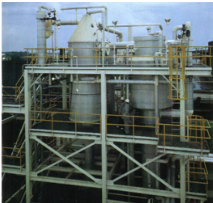
Forced-circulation thermal recompression crystallizer at the FMC Corporations Middleport, New York facility
