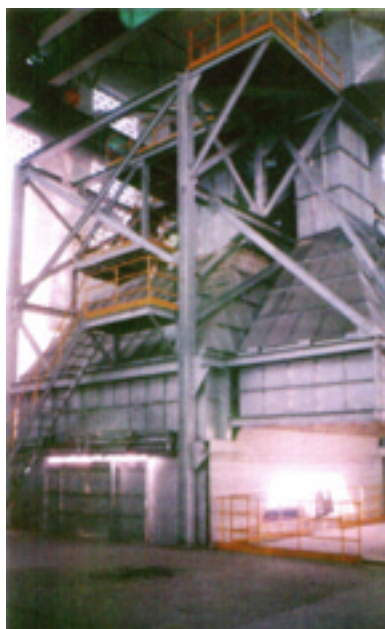
"Doghouse" style fume capture system employed on a 20-foot inner shell diameter arc furnace operation
