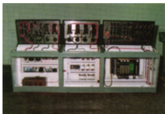
Console on left - with top panels raised for ease of maintenance
