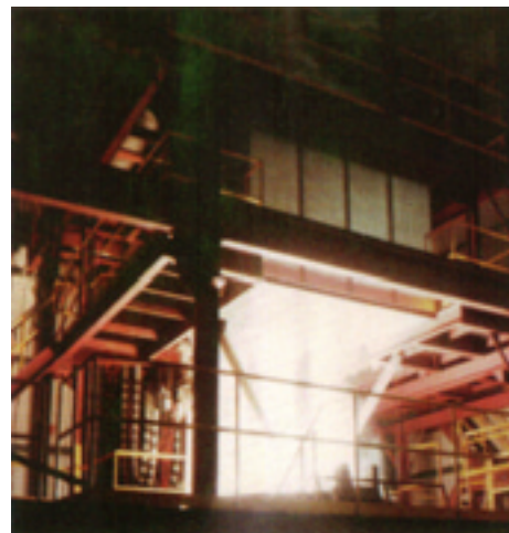
Canopy style fume capture system on a 10-foot inner shell diameter electric arc furnace application
