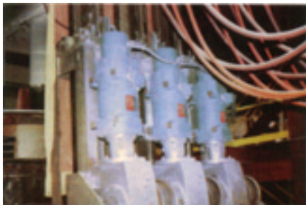
D.C. motor drives - An alternative to a servo valve type electrode mast positioner or as a retro-fit "upgrade" on older equipment.
