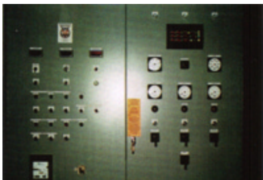
Custom built, electric arc furnace wallmount operator's control panel. Mineral fusion operation
