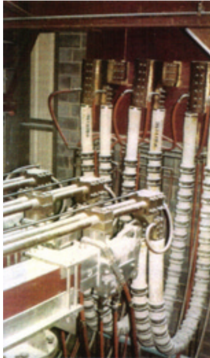
Water cooled electric arc furnace secondary components
