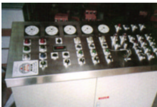
Custom built, electric arc furnace operator's control console. Steel scrap melting operation
