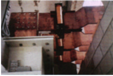
Furnace transformer secondary Delta closure assembly, air cooled design
