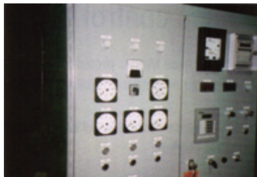
Microprocessor type, electric arc furnace wallmount operator's control panel. Mineral fusion operation
