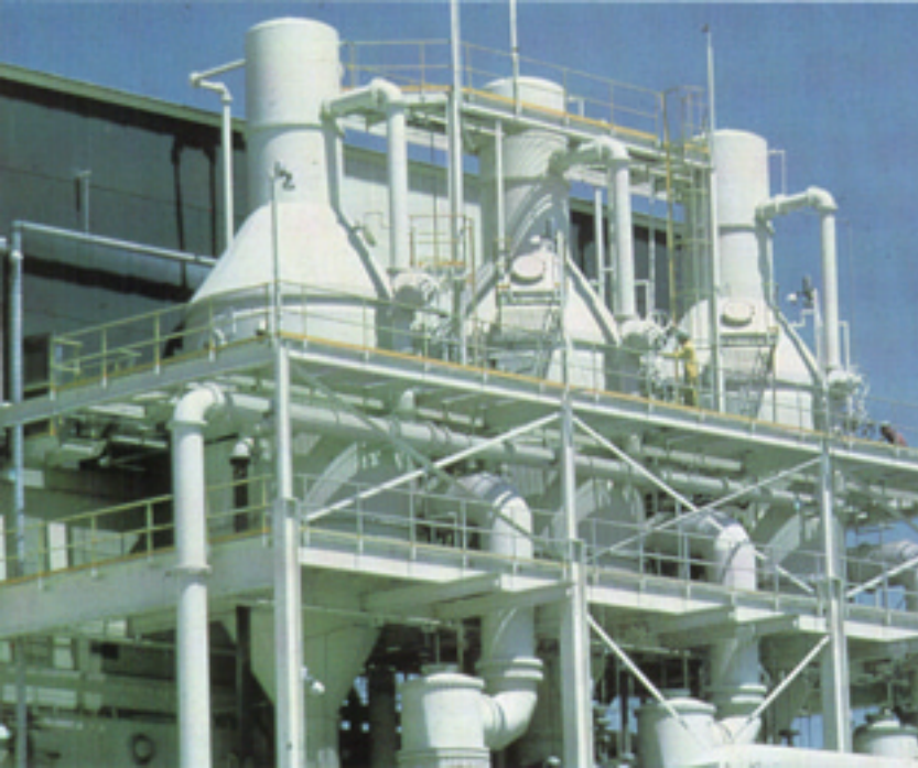
SWENSON three stage forced circulation evaporator.
