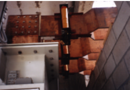
Furnace transformer secondary Delta closure assembly, air cooled design
