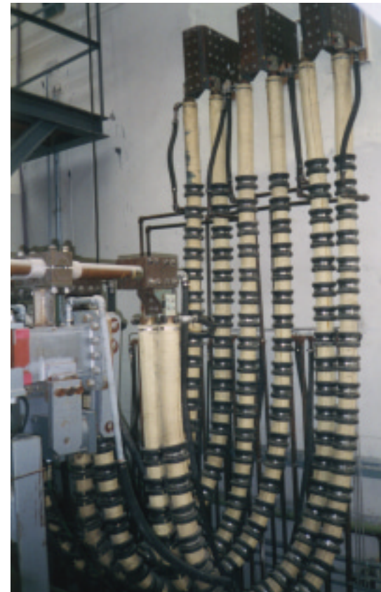
Water cooled electric arc furnace secondary components
